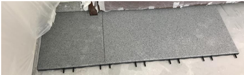
Installation of the tiles along a wall with the connector pins towards the next row
