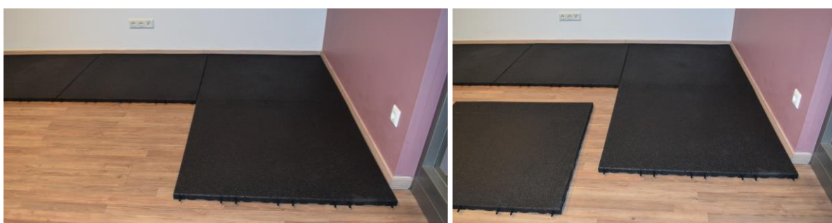
Start the second row of the tiles in the same way and continue; place the tiles next to each other
