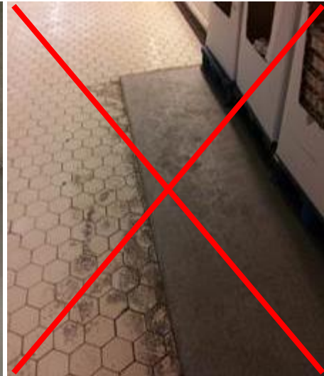
uneven, not suitable substrate
